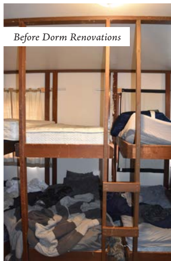
A glimpse at the cold air dorms before the summer 2023 renovations, which shows chipped wood structures and older mattresses.
